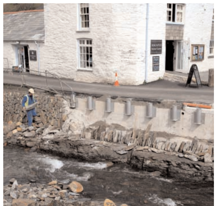
Below: Stonemasons at work on the facing wall by the Visitor Centre – timber bollards will be fitted into the galvanised steel sockets
