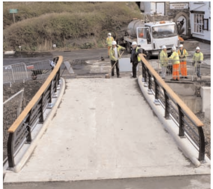
Above: Tarmac being laid on the roadway by the new Lower Bridge, which has now had oak handrails fitted
