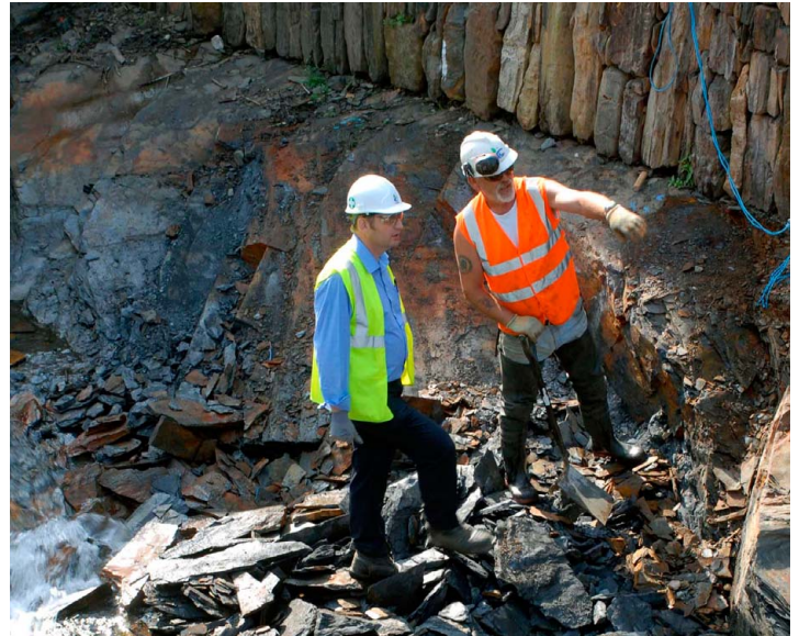
Above: Site manager Colin Mitchell with Stuart Lee who is clearing loose rock excavated under the main road bridge
